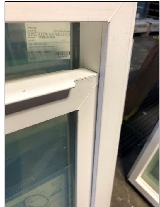
Both sides of sash in track (#2)
